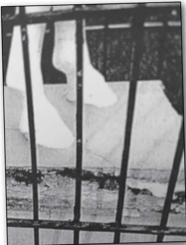
Corrosion built up over 20+ years Note the foundation and the rear portions of the front hooves.
